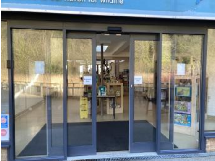
Automatic sliding entry door halfway open
